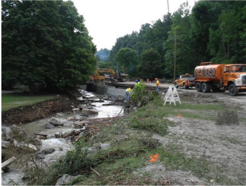
Repair crews working on extensive damage to Jamestown St. (Route 62) and the channel of Thatcher Brook (looking upstream) in the village of Gowanda.
